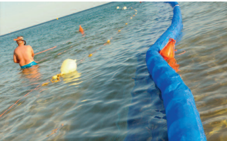
■ Each net is fixed with 'anchors with screws' up to three metres in depth, is 50m long by 25m wide and is put in place right along the beach
